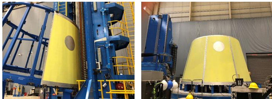
Figure 8. The Launch Vehicle Stage Adapter (LVSA) for the Artemis II flight is currently being welded at Marshall Space Flight Center (MSFC).
